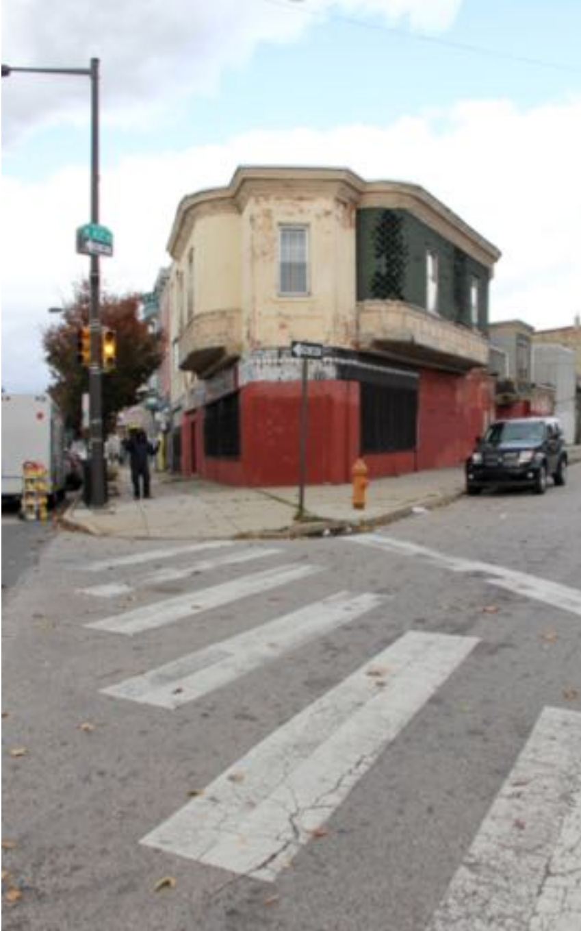
1 of 6 Corner Elevation, view to northwest. The original entrance of the second building that is currently sealed with bricks at the corner could be seen.
