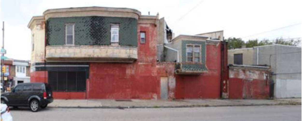
2 of 7 Elevation of northeast façade, view to southwest. Several alterations on the façade could be easily observed, including the sealed windows and entrance.
