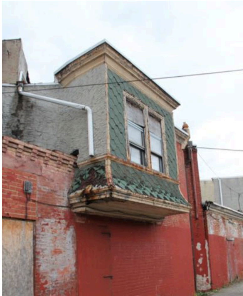
6 of 6 Photograph showing the addition of projecting bay covered by asphalt hexagon shingles in a bad condition.
